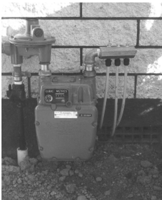
IPI system near gas meter
